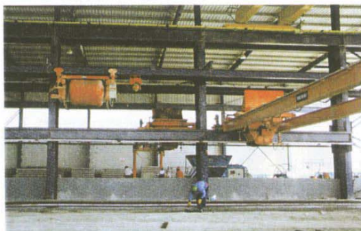
Fig. 3 Two frequency-controlled bucket rail systems feed the extruder via two half portals (one half portal per each part of the production hall).
