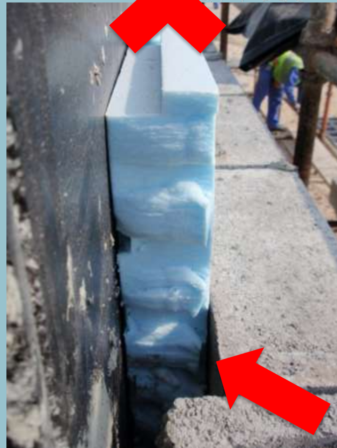
Gap in Insulation
