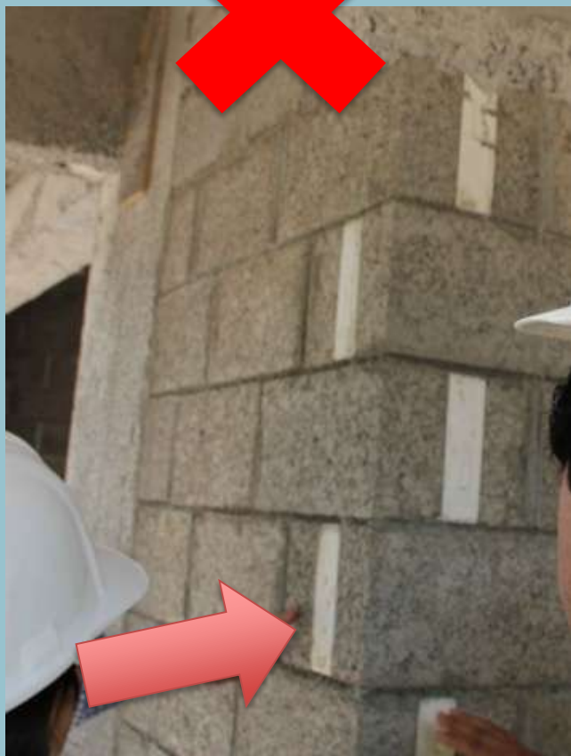
Incorrectly laid blocks / poor detailing
